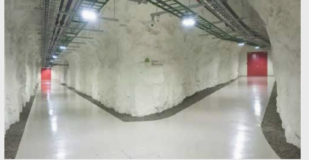
Görsel Kaynak: Amit (2022) Scan agrees partnership with Green Mountain Data Centres, Green Mountain Data Center. Available at: https://greenmountain.no/scan-partnership-hpc-services/ .
